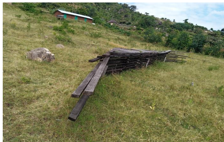
2. Roofing material left to warp
