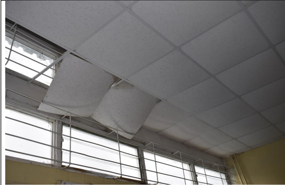
Falling pharmacy ceiling board
