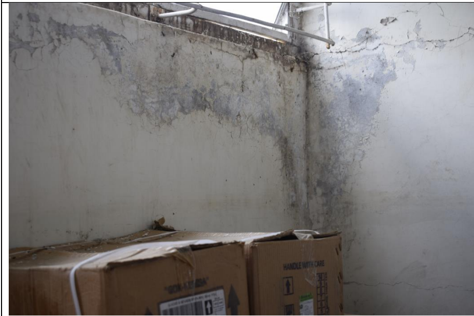
Pharmacy leaking roof
