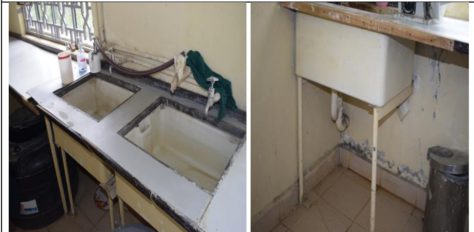
Sinks were not repaired
