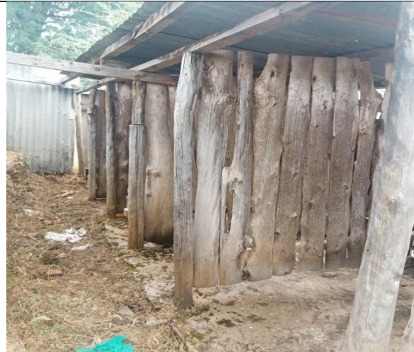
Figure 28: Females bathroom from inside
