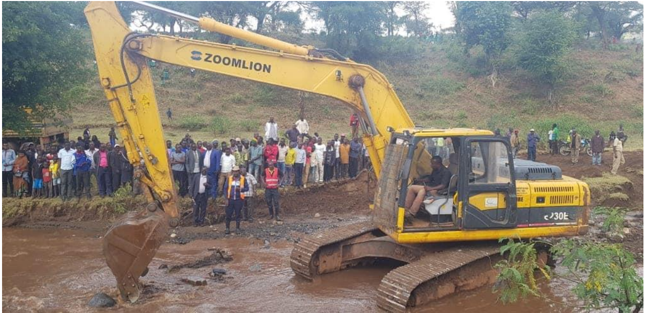
Figure 28: Roads department responding to Heavy rain cutting off Kitale-Kapenguria-Lodwar Highway at Ortum January 2020
